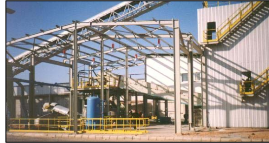
Batch plant detail
