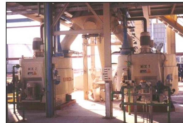
Batch plant: Mixers
