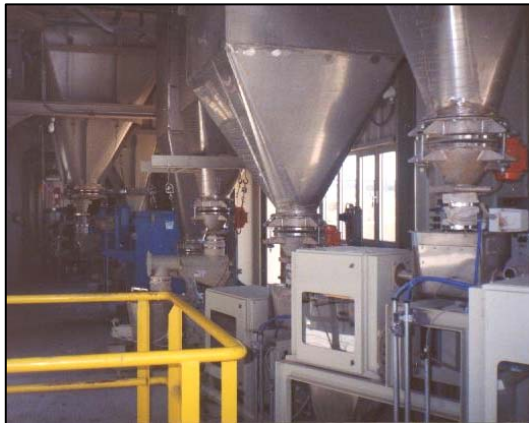
Batch plant: Additives silos and scales
