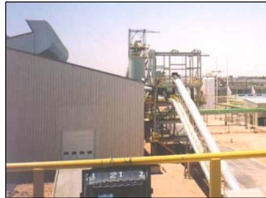
Batch conveyer stretching to furnace hall
